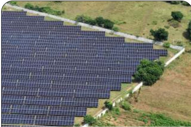
Solar Ground Mount
